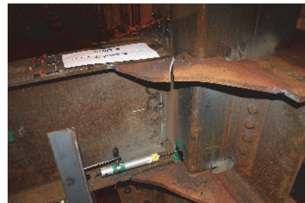
Fig. 13. HBC-3 (failure at upper diaphragm during 0.04rad)
