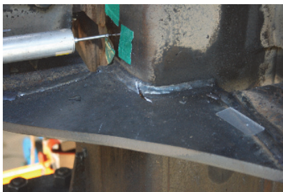
Fig. 11. HBC-1 (cracking at lower diaphragm during 0.05rad)
