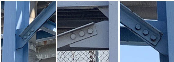
Fig. 1. Non-seismically detailed gusset plates welded to a column web only in pipeline supporting braced frames
