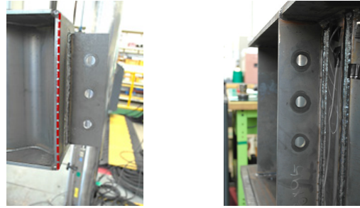
(a) Bending deformation of the end plate of beam comprising the FF-C (b) Bearing deformation observed in bolt holes of FF-C girder
