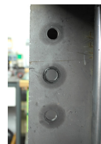
(d) Bearing deformation observed in bolt holes of PE girder
