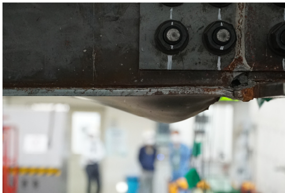
Fig. 9. Failure shape of HF-SRC-BR
