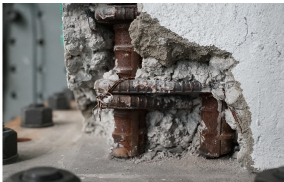
Fig. 13. Failure shape of HF-RC-BM
