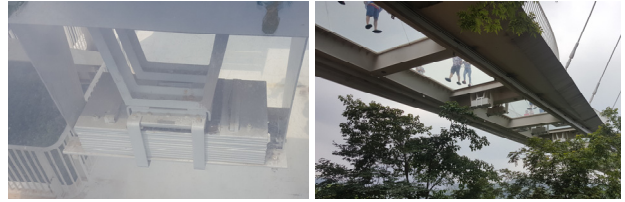
Fig. 4. Damping and anti-vibration system (China)
