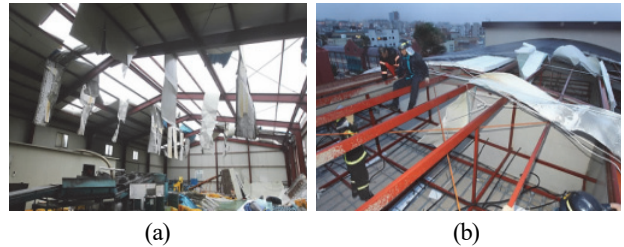
Fig. 3. Typhoons damage cases
