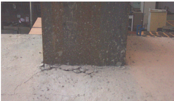
Fig. 11. Crushing of concrete slab of PN700-C at 3% story drift
