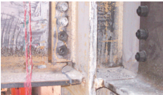
Fig. 10. Beam bottom flange fracture of PN700-C at 3% story drift
