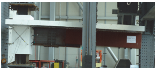
(b) W/ connection reinforcement; GCR04
