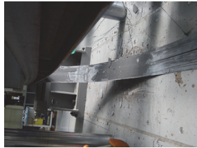
(c) CFRP debonding (Final, B4C1.4F)
