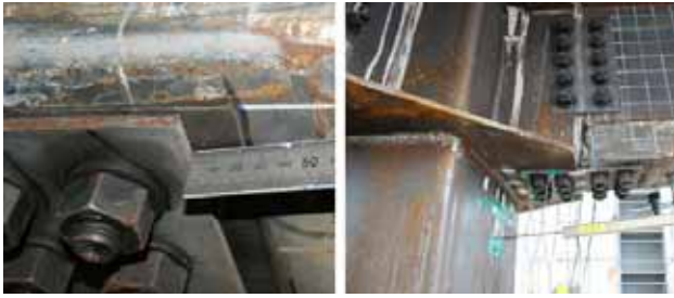
Fig. 17 Failure Shape of HF5-A-8 specimen : Slip and Bearing Failure
