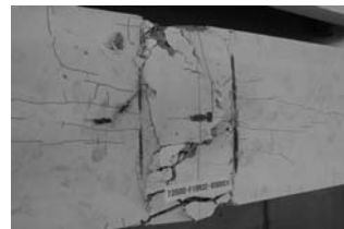
Fig. 13 Failure shape : no bottom rebar
